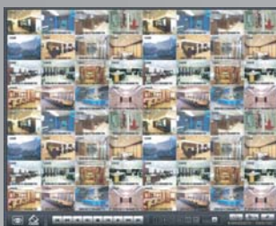
central monitoring system (CMS)
